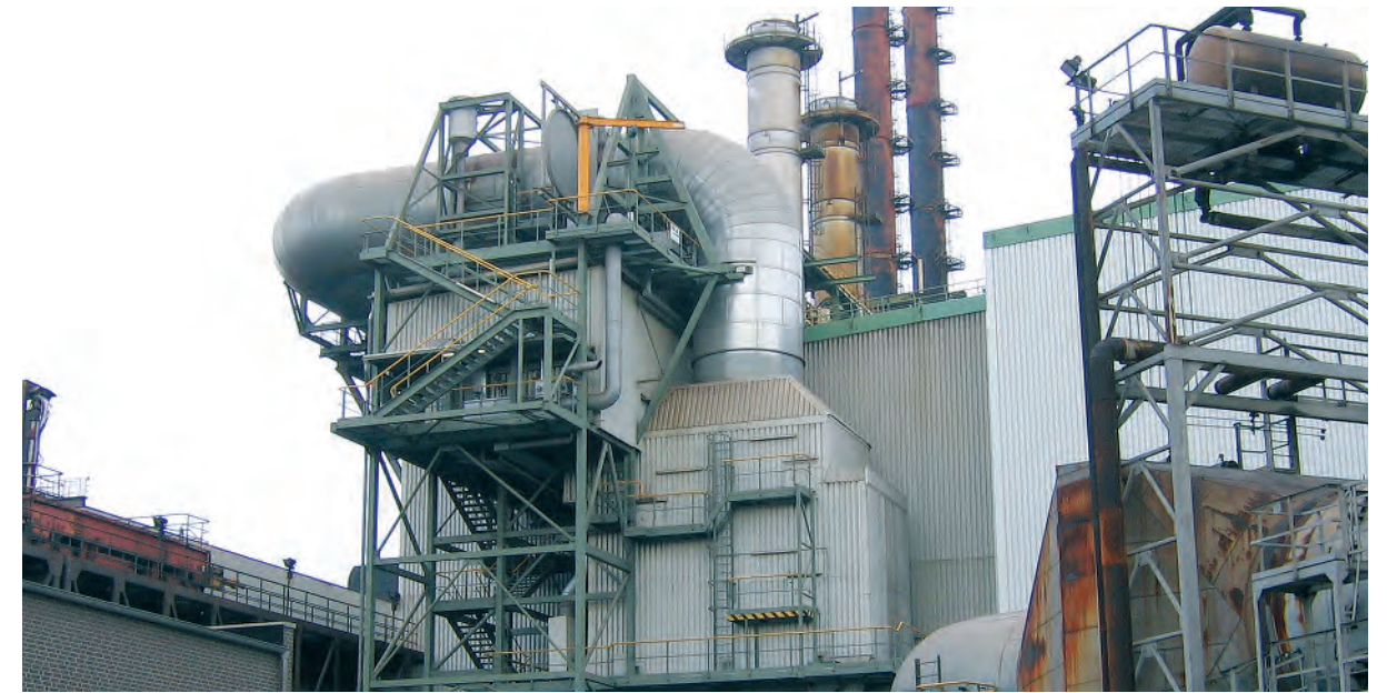
Waste heat recovery in downstream pusher-type/walking beam furnaces
